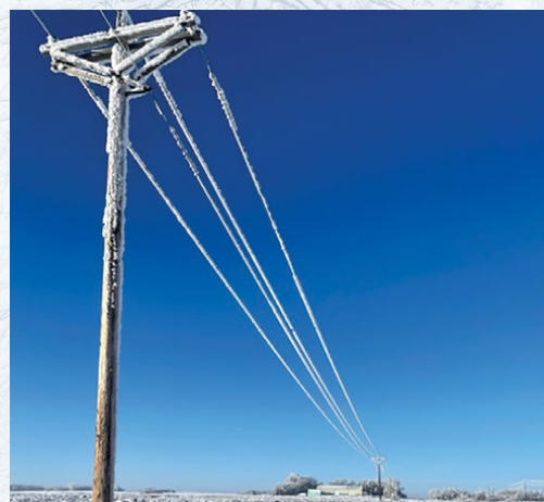
Ice that accumulates on lines and strong, high winds can impact distribution.
