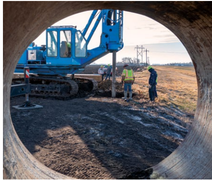
A 20-foot hole is bored to hold a new laminated power pole near Walle substation.
