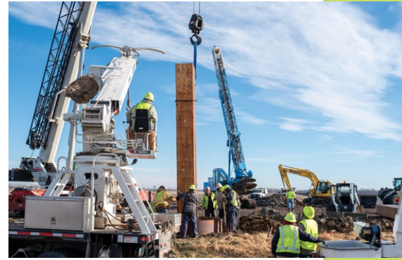
Crews use a large crane to lift the structure into the bored hole.
