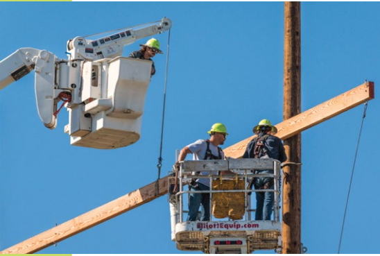
Minnkota's line crew works together to reroute a 230-kV line around Walle substation.
